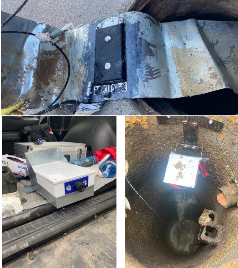
Slika 4. Gore) Elektromagnetni sensor na nosećem limu nakon demontaže; Levo) Kamera pre montaže; Desno) Montirana kamera na mernom mestu Figure 5 Above: Electromagnetic flat sensor on metal sheet support after deinstallation. Bottom left: NIR camera before installation, Bottom right: NIR camera in installed position
