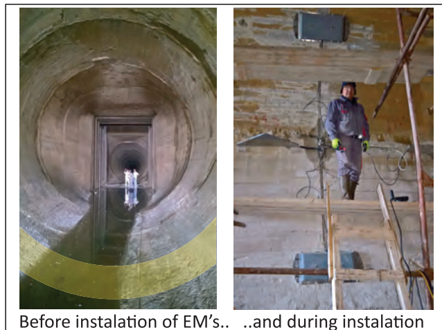
Before instalation of EM's.. ..and during instalation Figure 20. F-B tunnel, inlet cross section F-B IN before installation of equipment (left) and during the installation (right)
